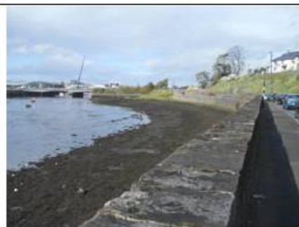
Raised wall of right bank of Garavoge River downstream of Hyde Bridge
