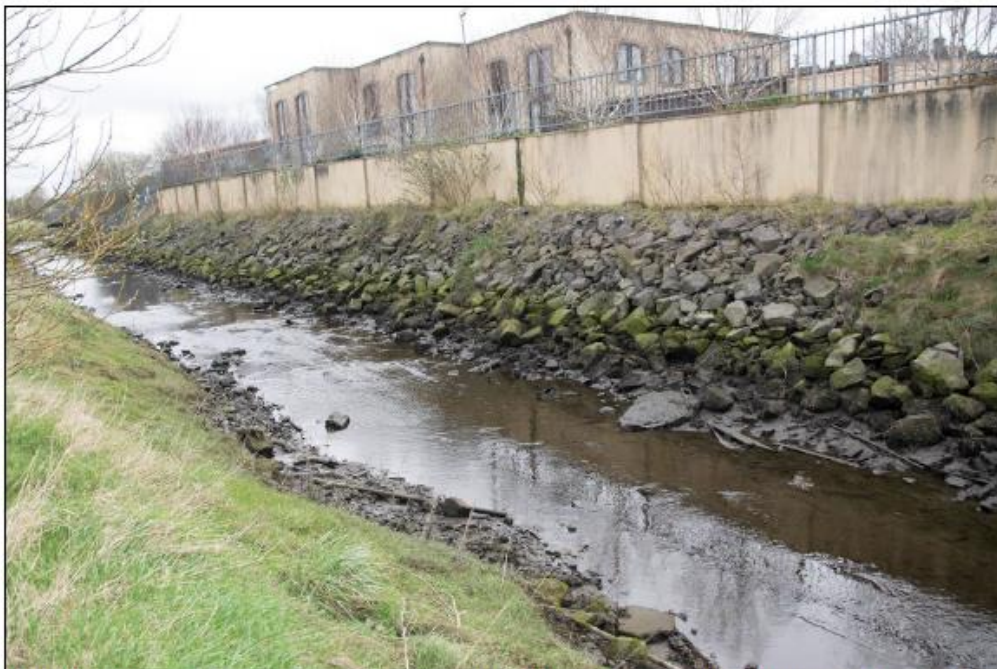
Plate 6 Stretch of the Copper River approximately 100m upstream of the N4 Bridge. This part of the river is influenced by the tide.
